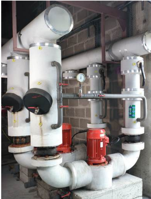
Example of using the Altistart 22 soft start/soft stop unit in a pumping application
